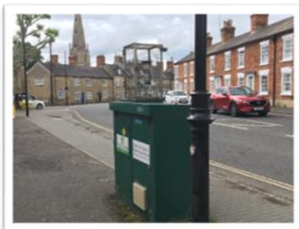
Roadbox 2 Monitoring Station High Street South, Olney
