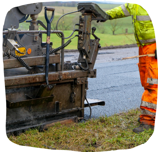
An asphalt paver machine laying new asphalt onto a road. The highways operative controls the distribution of the hot material using a control panel. After this, it is compacted and finally rolled to ensure a smooth, set surface.
