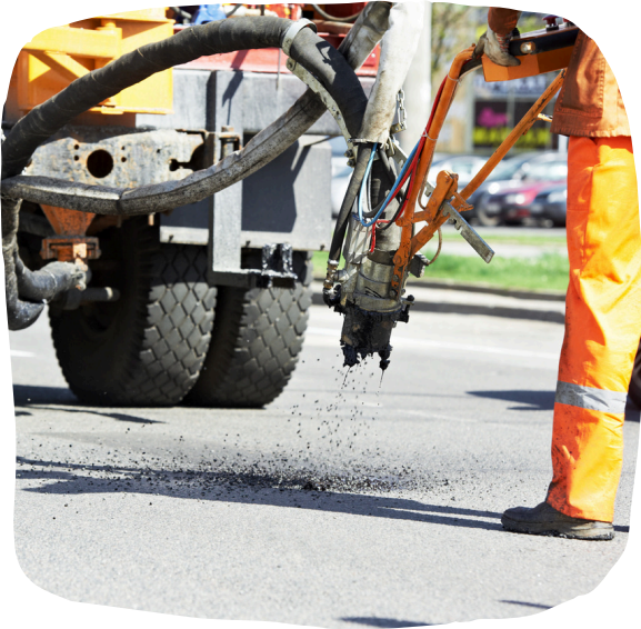
A spray injection machine filling a road defect with a mix of small stones and bitumen.
