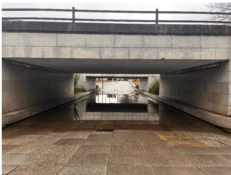
Figure 19: Flooded underpass in Central Milton Keynes. Source: shared directly from Milton Keynes City Council.
