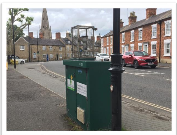
Roadbox 2 Monitoring Station High Street South, Olney
