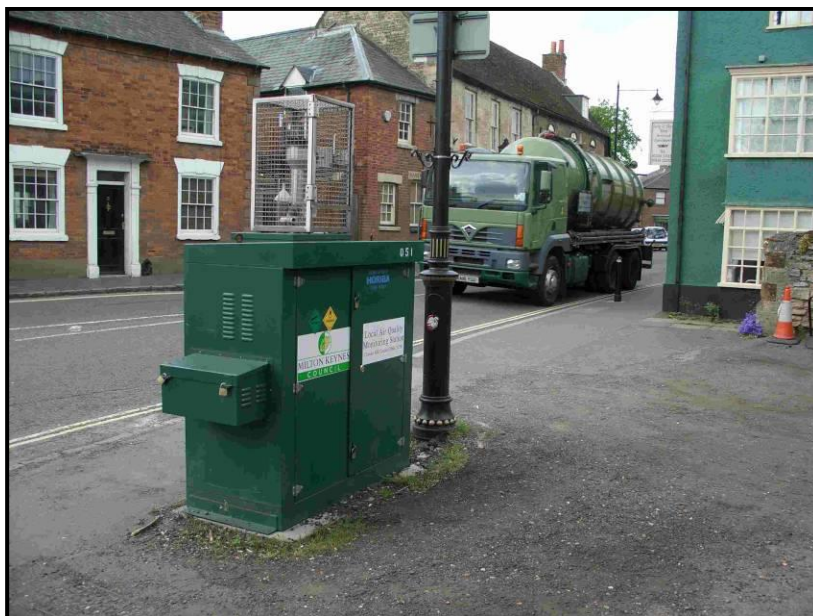
Figure 2 Olney Air Quality Monitoring Station
