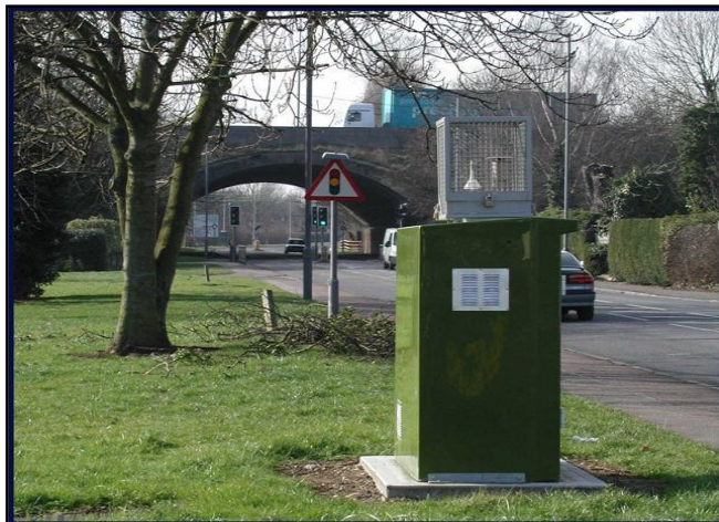
Roadbox 1 Monitoring Station Wolverton Road, Newport Pagnell (M1 bridge in background)
