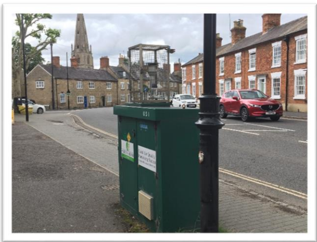
Roadbox 2 Monitoring Station High Street South, Olney
