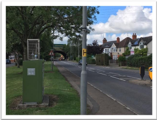
Roadbox 1 Monitoring Station Wolverton Road, Newport Pagnell (M1 bridge in background)
