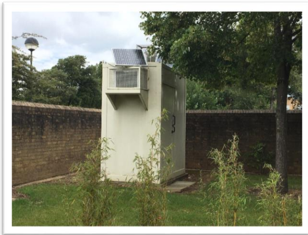
Static Monitoring Station, Civic, CMK.
