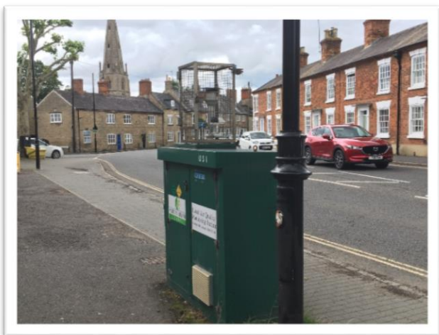
Roadbox 2 Monitoring Station High Street South, Olney
