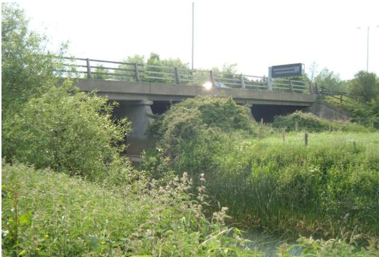
Figure 8 - River Ouzel beneath the M1, showing tie into highway embankment (downstream – left bank)
