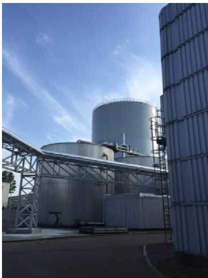
The new heat storage system at the city of Dessau-Roßlau.
