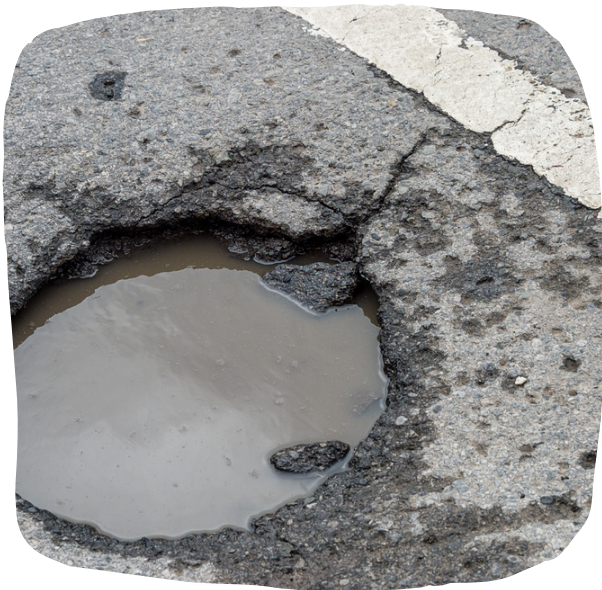
Example of a 'deep pothole'. It has a sharp-edged hole in the top road surface layer.
