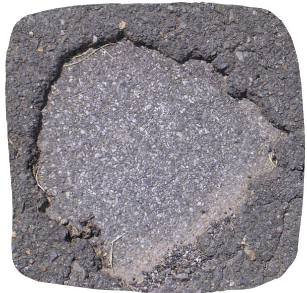
Example of a 'shallow pothole'. It is much lower in depth.
